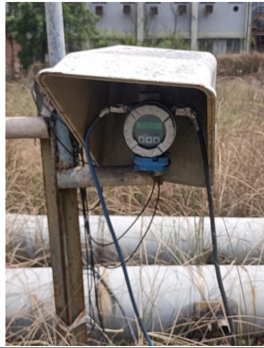
CT Blowdown Flow Meter
