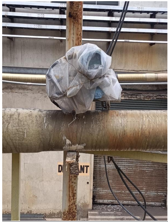
SW RO Flow Meter
