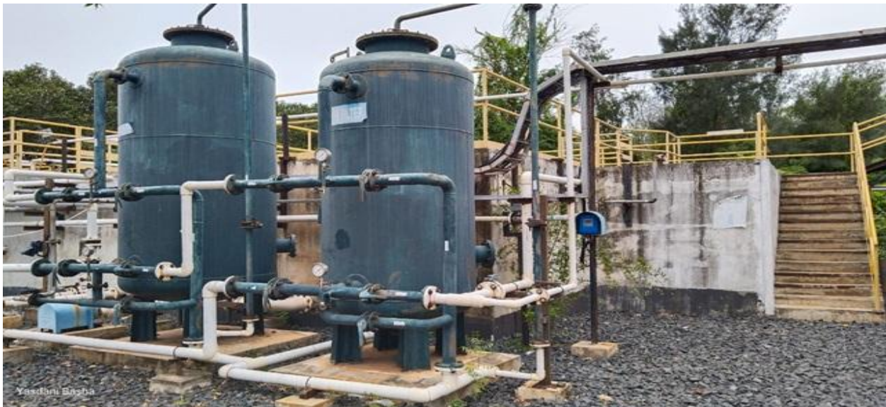
Sewage Treatment Plant
